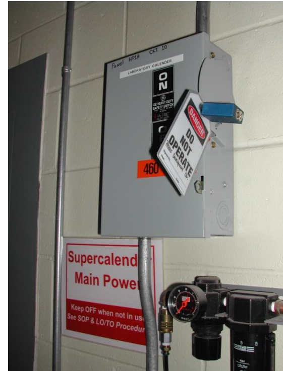
Lock Out tags on various pieces of equipment.
