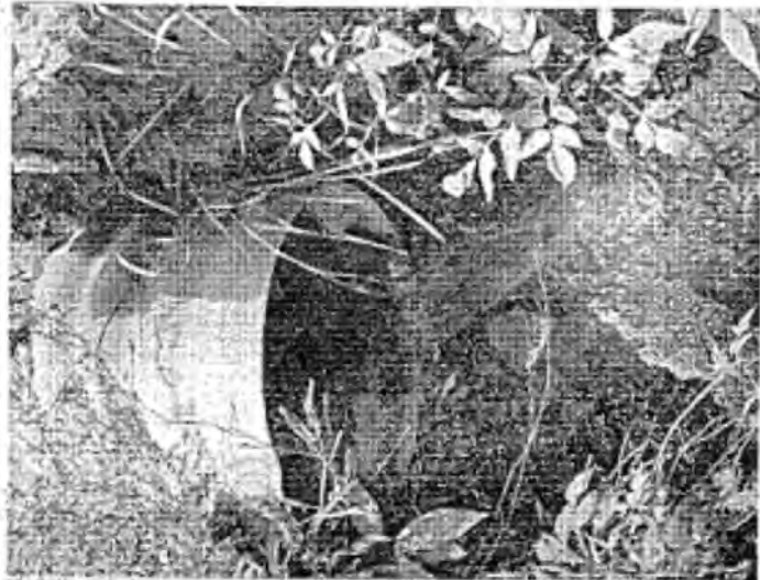
ALMOST HIDDEN CULVERT disgorges polluted water into the beautiful and popular Saco River in the area of Conway Village. Pollution sources such as this will be cleaned up when Conway installs its long-awaited disposal system. (Photo by Jay Hanlon)
