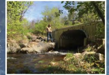
Mill Creek passes through a restored "ironstone culvert" built beneath the road to Pierce's Pond.
