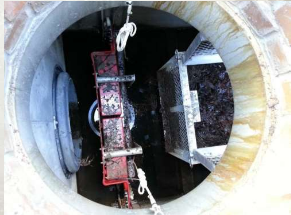
Broadway Street – Outlet Control Structure Inside NSBB
