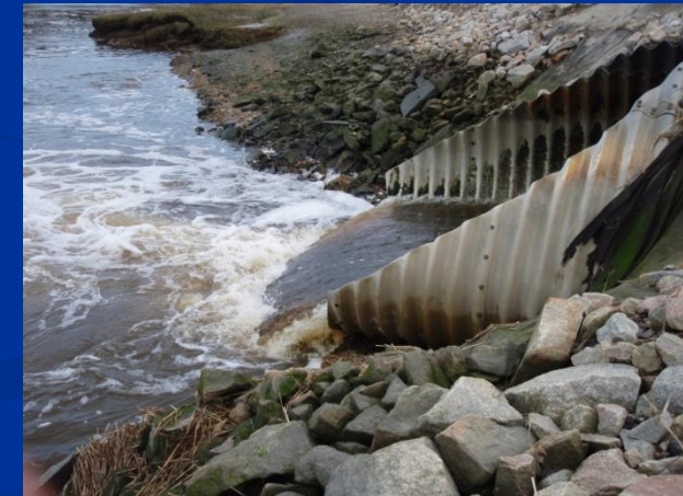
Hanging Culvert, Cascade Brook, ME
